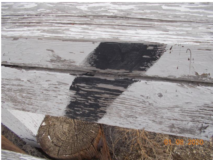
Paint sample M-22-Y-LP02. The black paint is considered lead containing paint.
