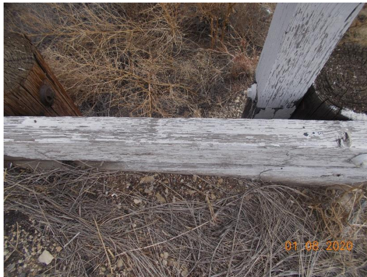
Paint sample M-22-Y-LP01. The white paint is considered lead-based paint.
